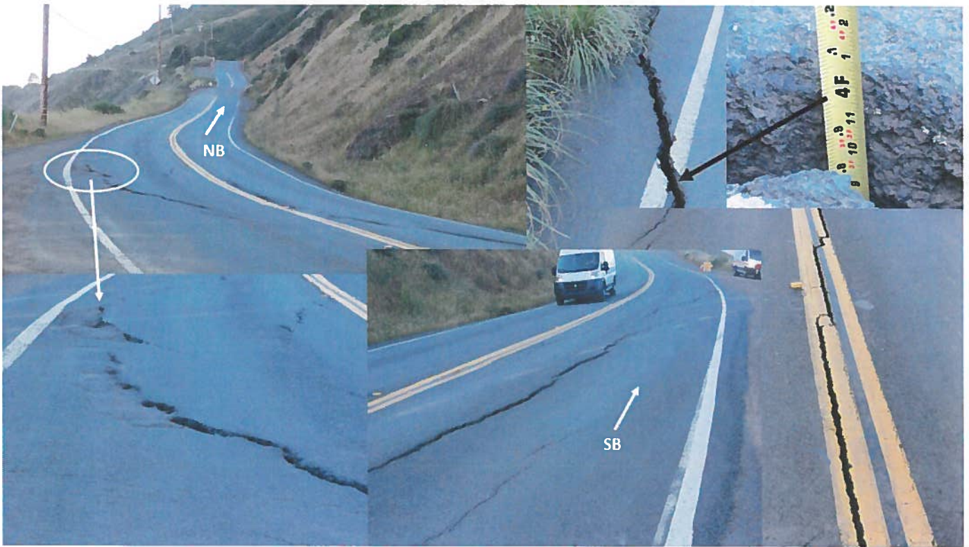
Significant cracking and settlement in the roadway throughout the damaged section of roadway
