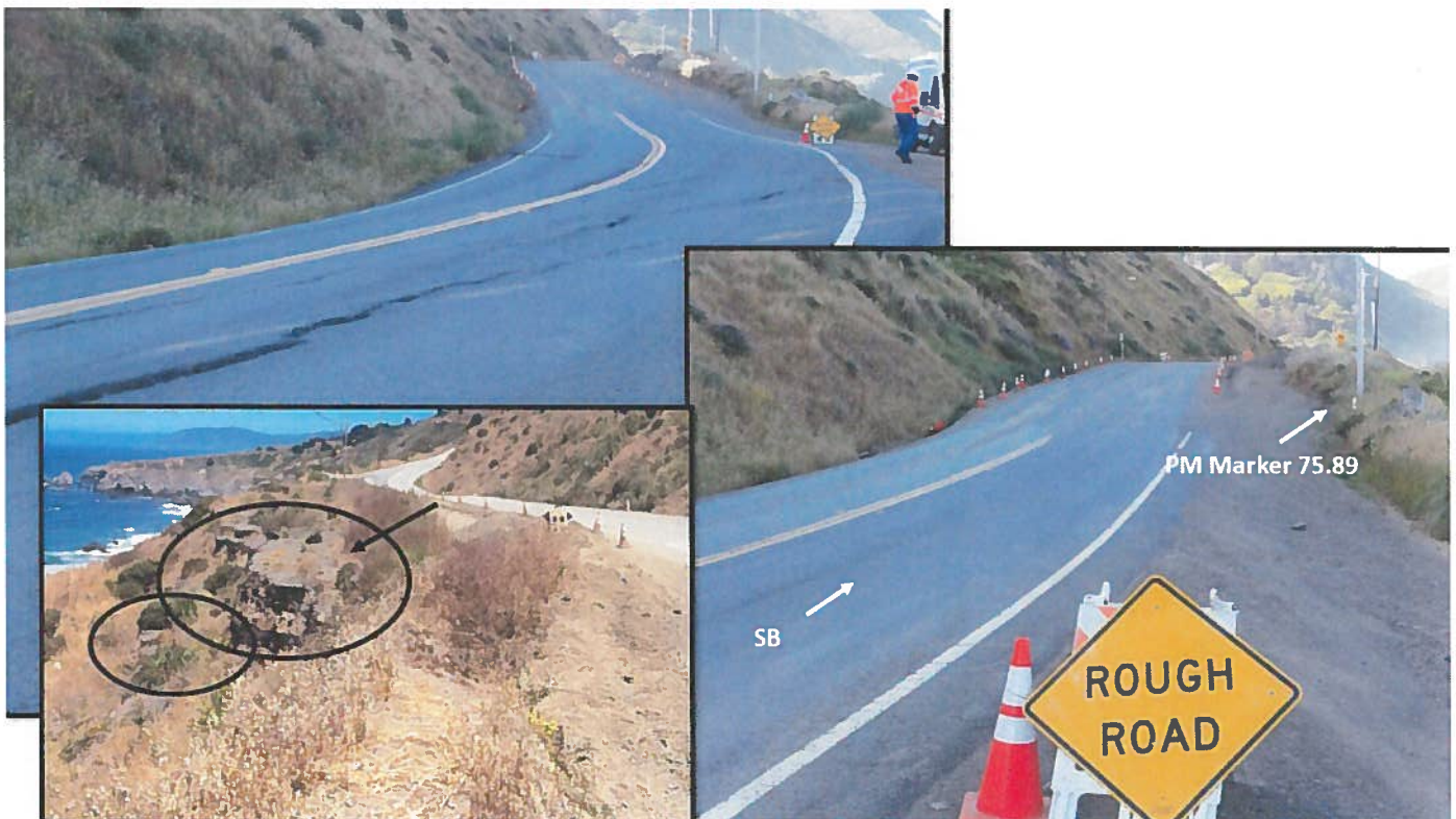
Southern section of the roadway (note encircled areas show historic and recent settlement of shoulder)
