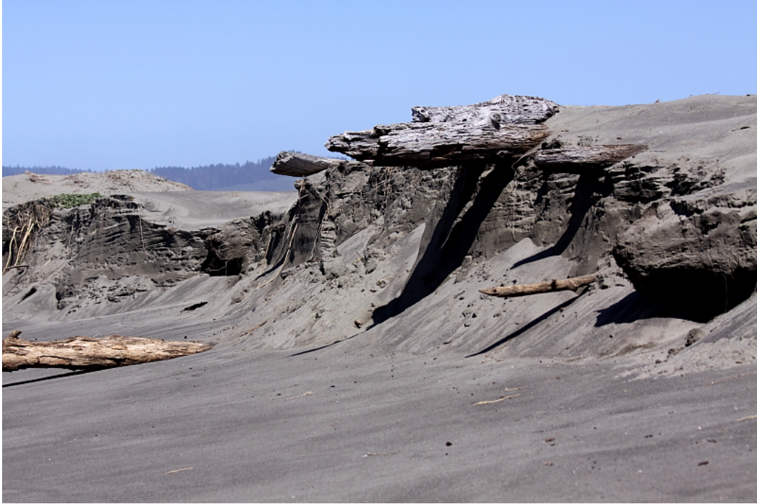
Crumbling portion of old Haul Road within the Natural Preserve. April 2010.
