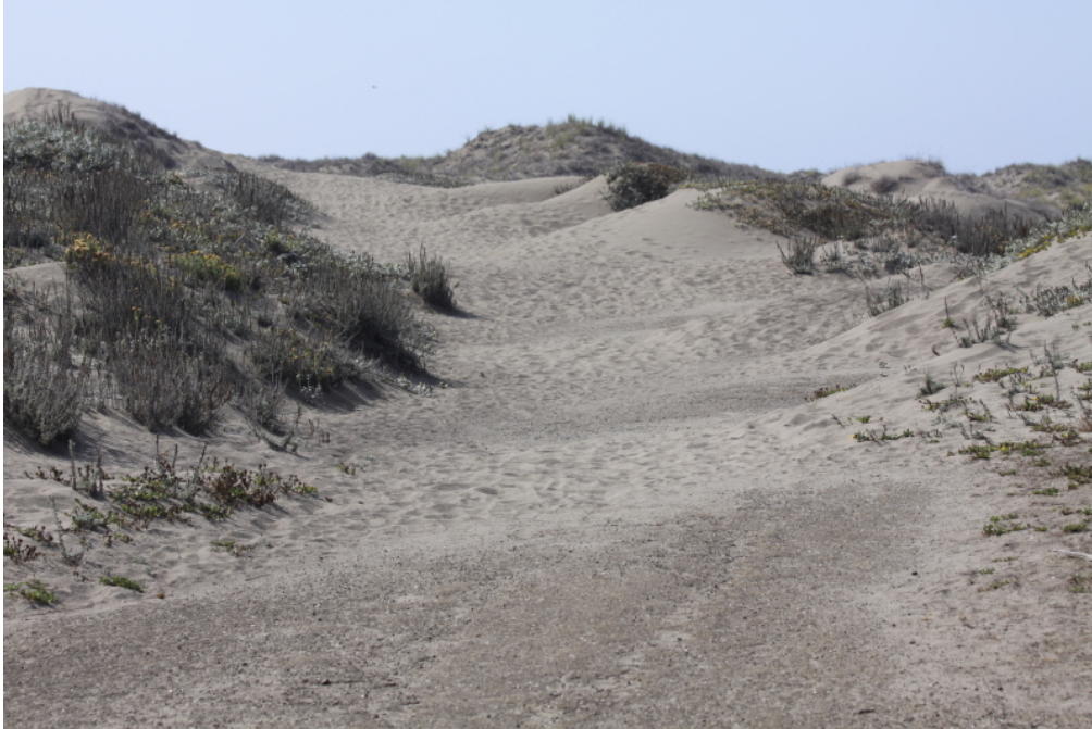
Portion of the Haul Road approximately 200+ feet in length where the road is completely covered in sand up to 3 feet deep. September 2009.
