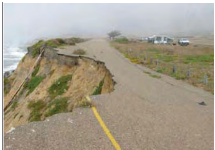
Bluff erosion on old highway near Abalone Point.
